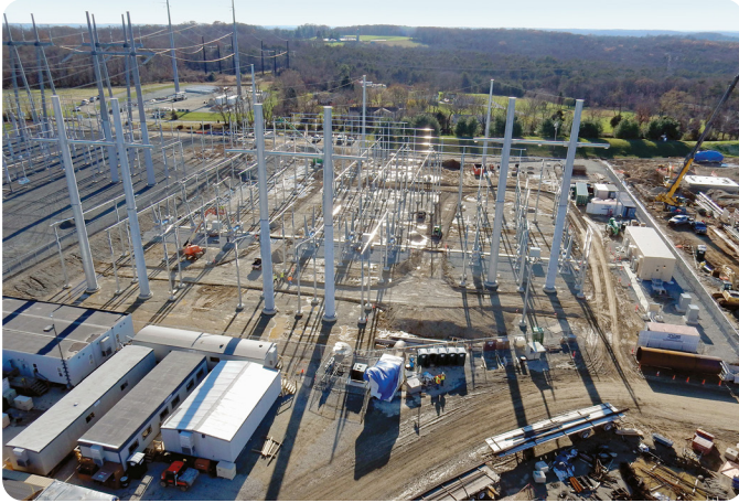
Wildcat Point Generation Plant
